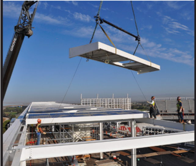
Cupertino Electric (No. 19) designed and built all the electrical infrastructure for Levi's Stadium, home of the San Francisco 49ers NFL football team, in Santa Clara, Calif. It opened in July. The work included a 49-panel solar installation (see above).
